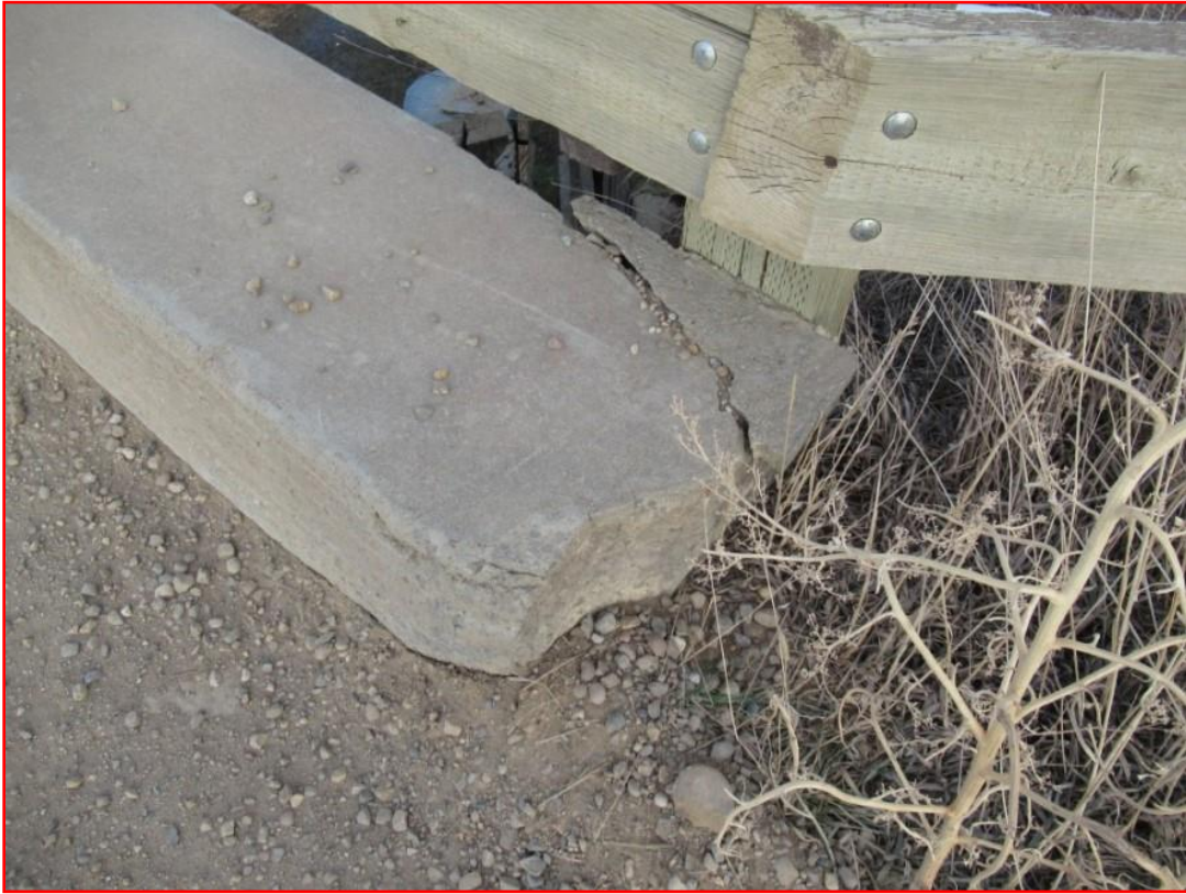
Photo 5: Curb Spall on SE Corner
