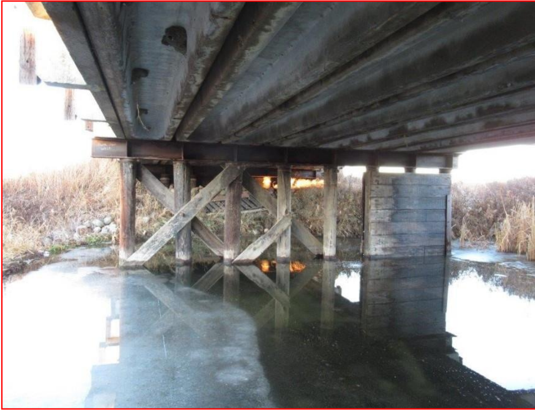
Photo 3: North Pier (P2) Nose Plate Requires Fastening
