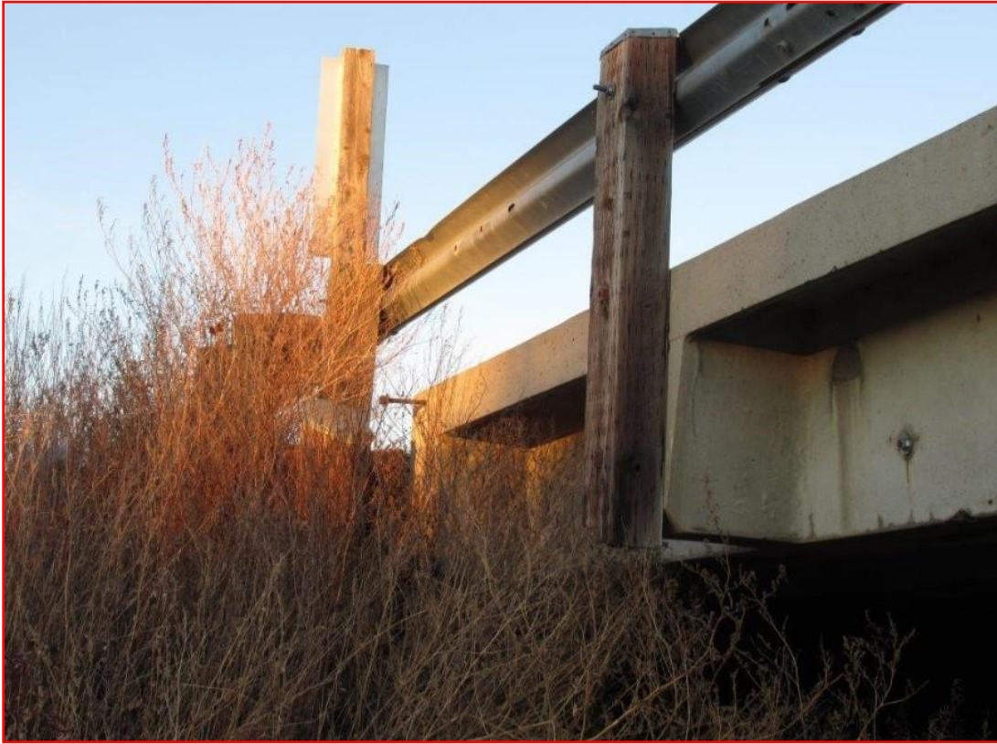
Photo 1: Missing Timber Rail Post
