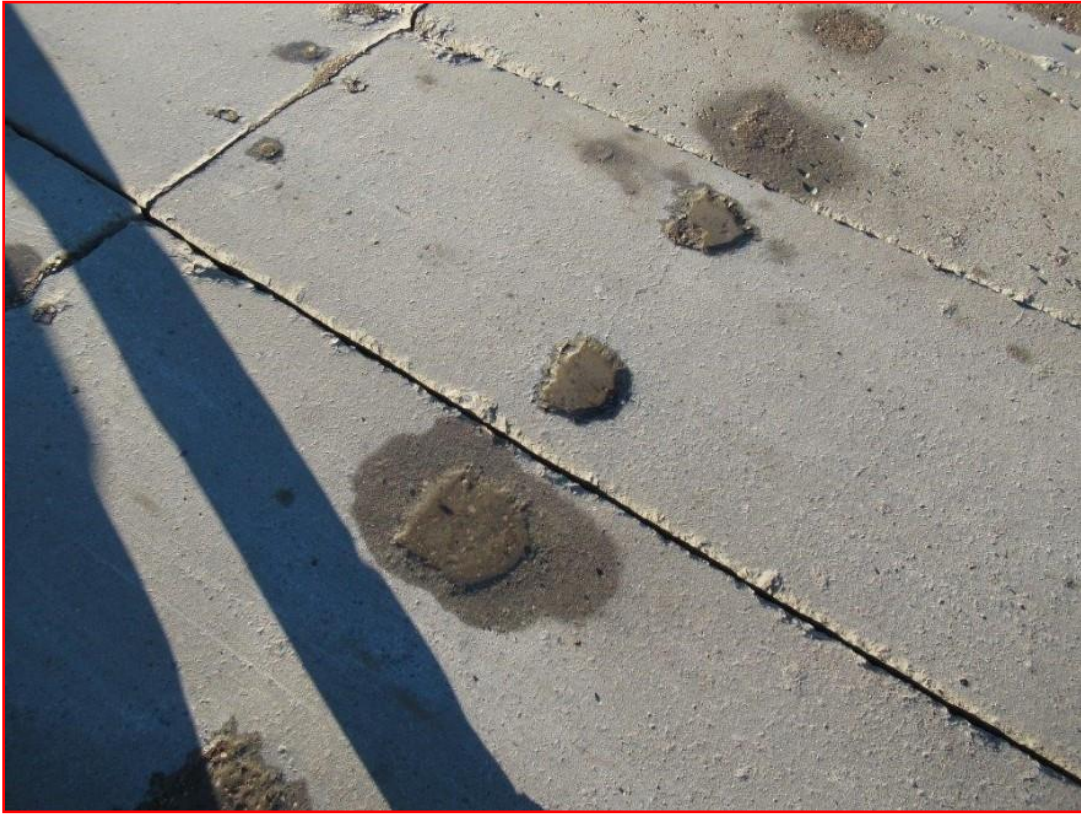
Photo 1: Girder Lift Pockets full of ice
