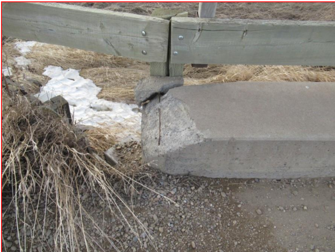
Photo 4: Curb Spall on SW Corner affecting anchorage (Concrete Repair)
