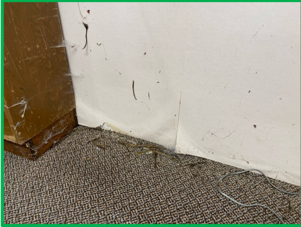
Water Staining / Water Damage
